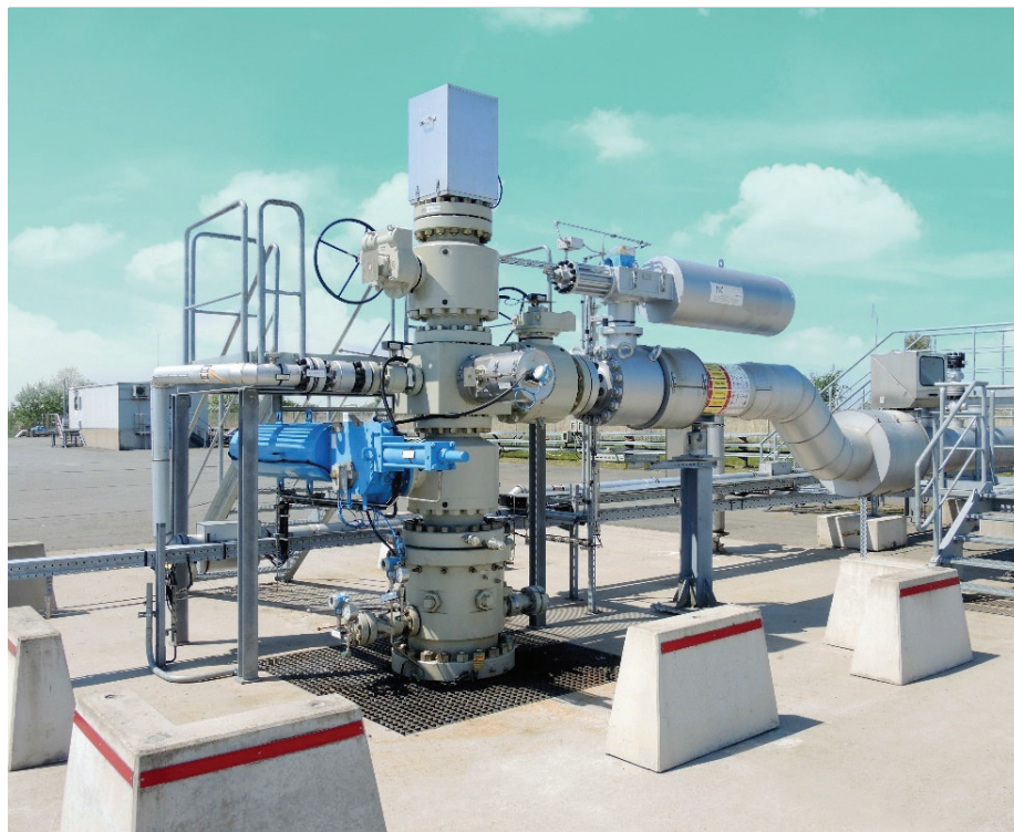
Fig. 2 Gas cavern well head – state of the art
