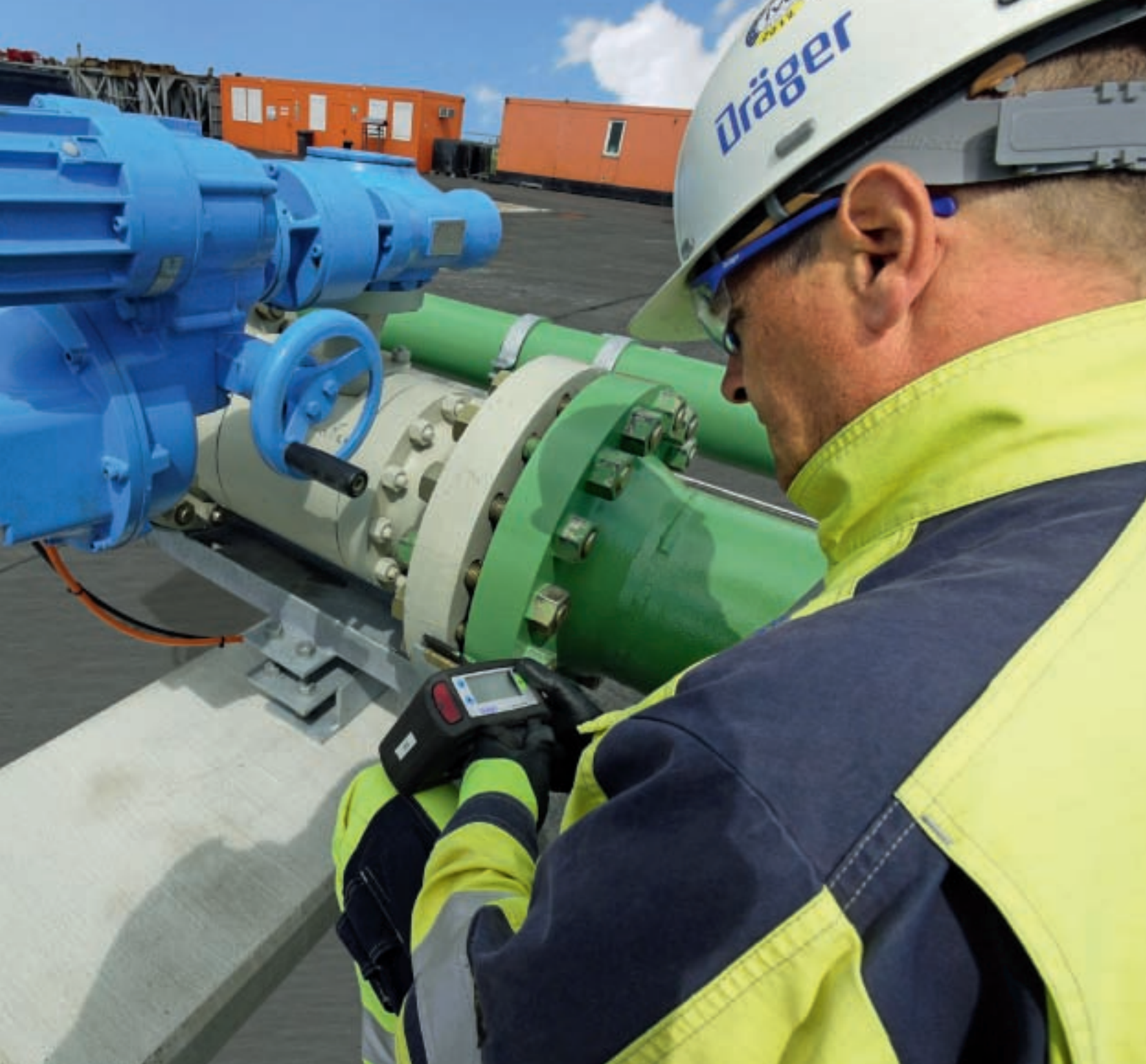
Safety first: Bernhard Hamphoff from Dräger measures a pipe flange to ensure there are no gas leaks.
