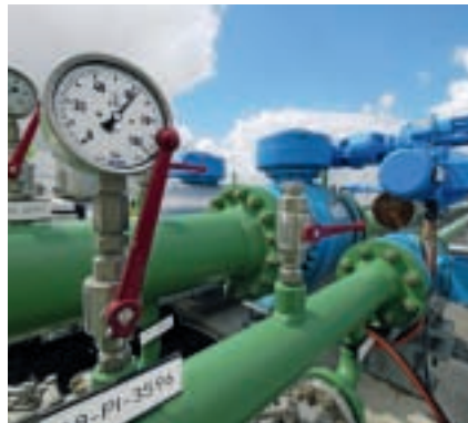
Pipes, valves, and pressure gauges hold the gas in check.
