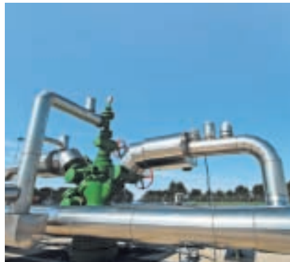
Piping is the only sign of the cavern many meters underground.
